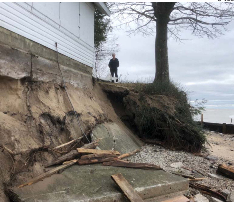
EIGHTEEN METERS OF BEACH lay in front of Ron Wilson's cottage on Lake Michigan as recently as 2013. Last fall, the lake was lapping at the cottage's structure.
